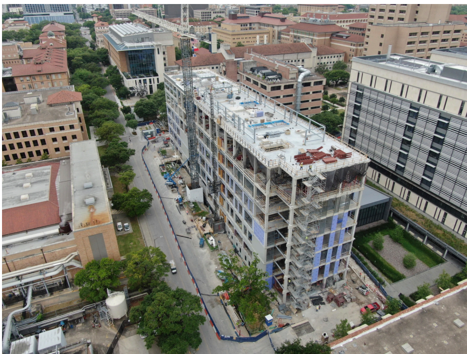
Aerial view of construction site for the new Gary L. Thomas Energy Engineering Building.
